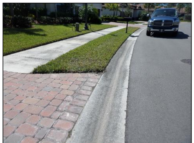
Water stains/chips at gutter – south area
