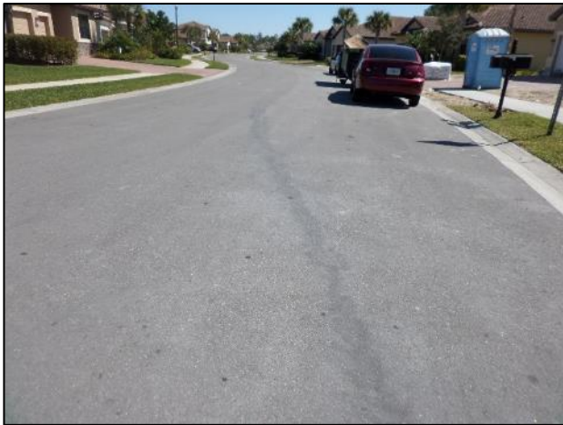
Stains in roadway surface – south area
