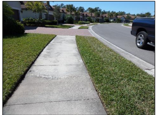
Stains on concrete sidewalk - south area
