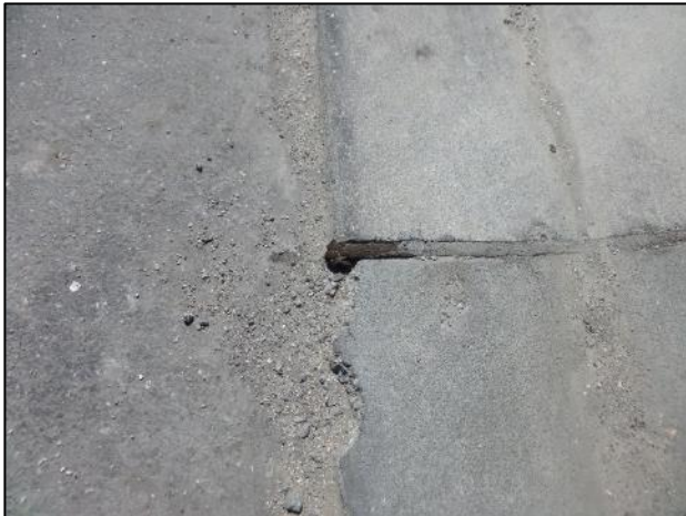
Chipped gutter – north area
