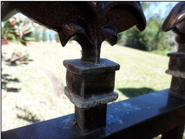
Deterioration/oxidation at decorative fence
