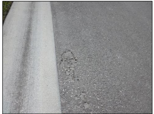
Sporadic gauges in roadway surface - north area
