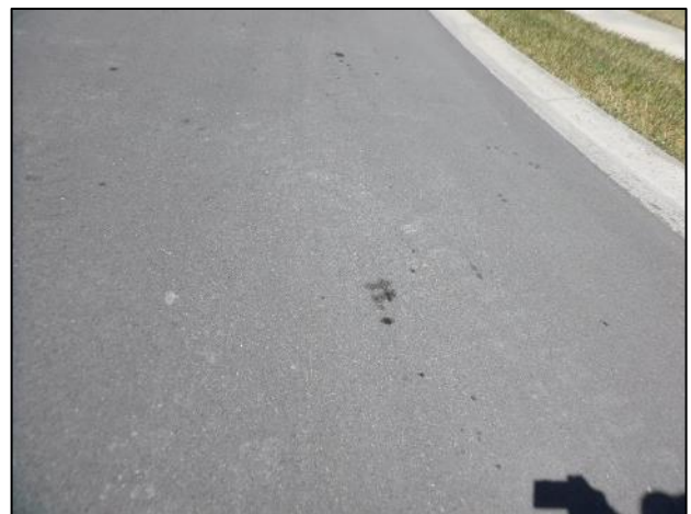
Stains in roadway surface – south area
