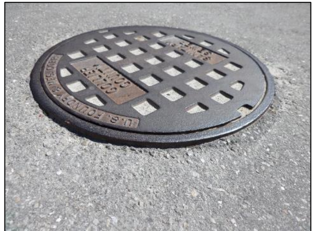
Final asphalt lift needed at north area
