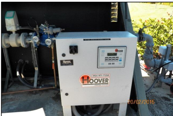
Variable Frequency Pump control
