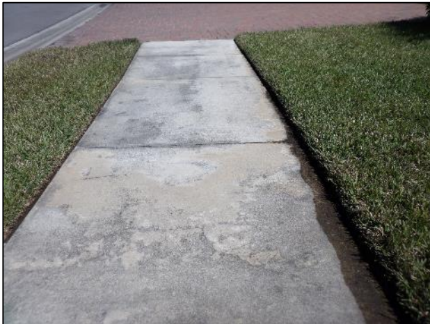
Stains on concrete sidewalk - south area
