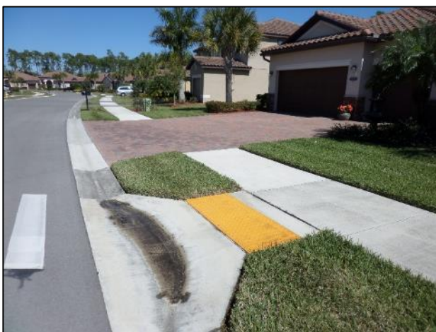
Stains on concrete walkway – north area
