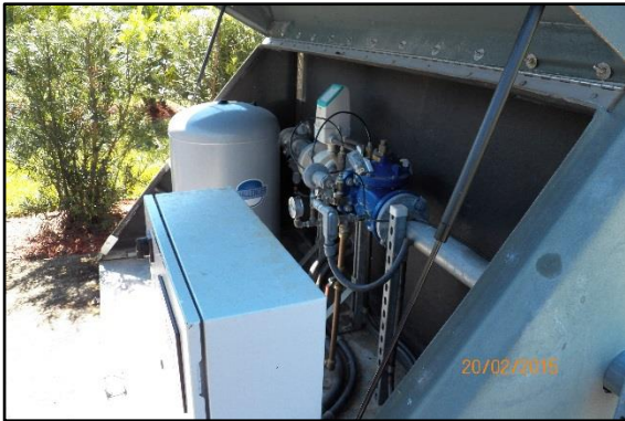
Dry components of the pump station
