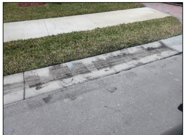
Gutter stains at north area
