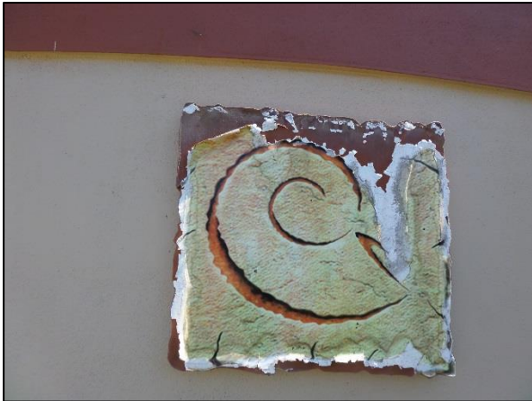
Main entrance sign decal deterioration
