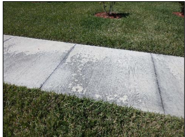
Stains on concrete sidewalk - south area
