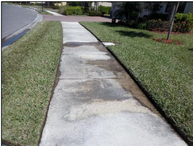
Stains/standing water on concrete sidewalk
