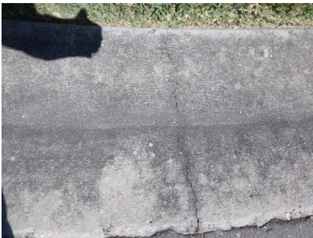
Gutter stain/chips at north area
