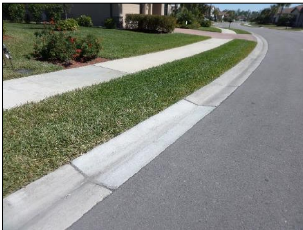
Evidence of repair of concrete gutter – south area
