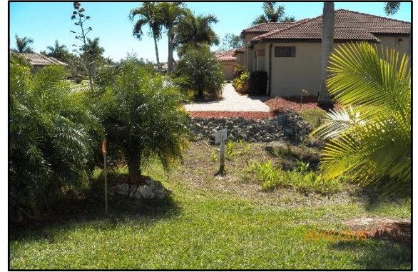
Encroaching Retaining Wall in Preserve
