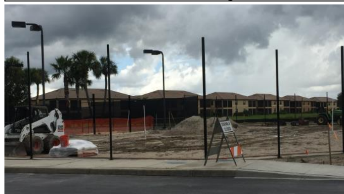
Final construction on Court 9 is expected to be completed by October 31th.
