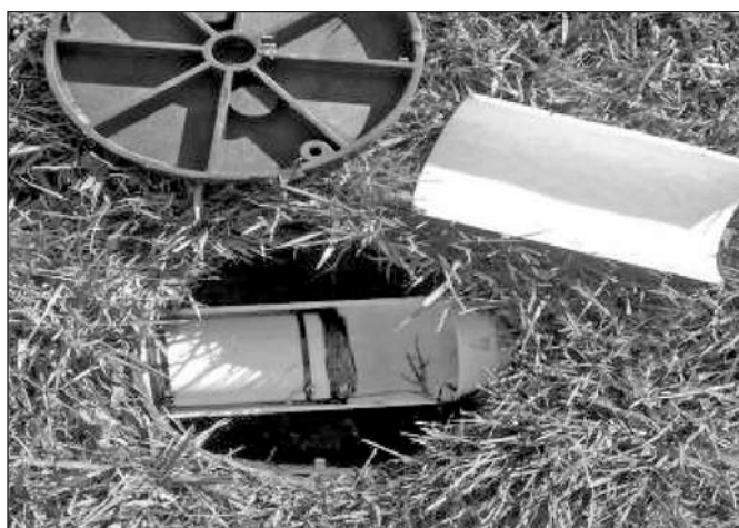
Figure 2 Filter cartridge inserted into filter housing, all within an easily accessed irrigation box.
